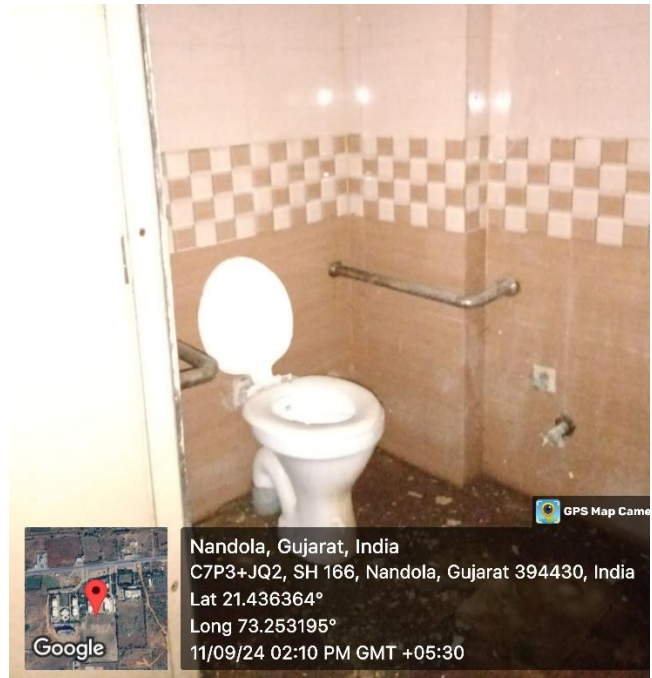
Disable friendly washroom
